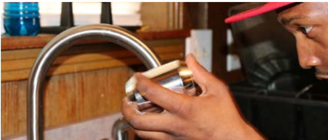
People's Advocacy Institute member installing a water filtration device at a residence in Jackson, Mississippi.
